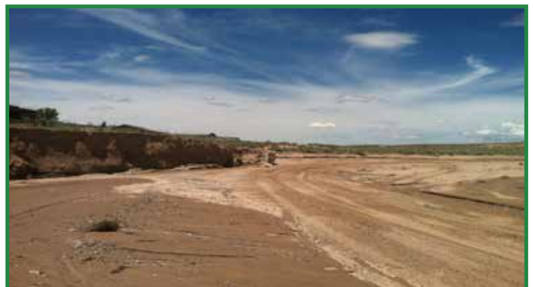
Bank erosion threatening infrastructure
