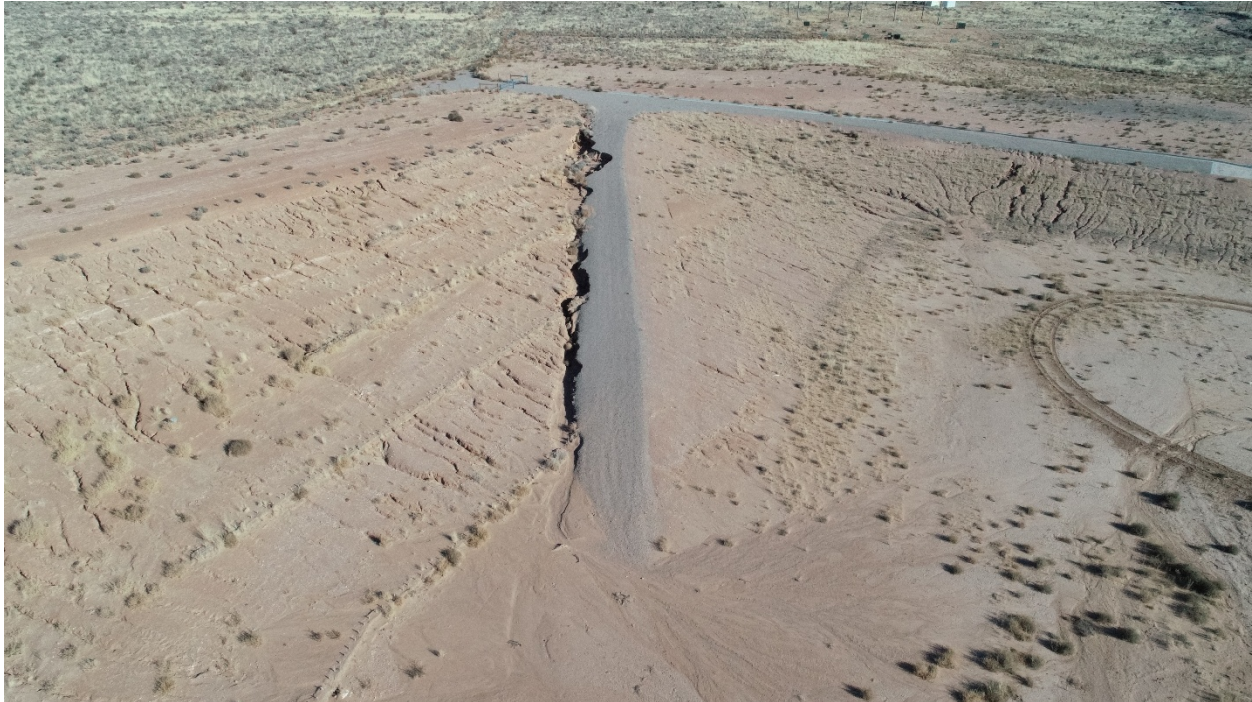
Figure 2 Channel degradation & damaged maintenance access ramp.
